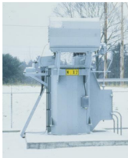
Plate 5.12 – Typical Auxiliary Power System Image: ©ABB
