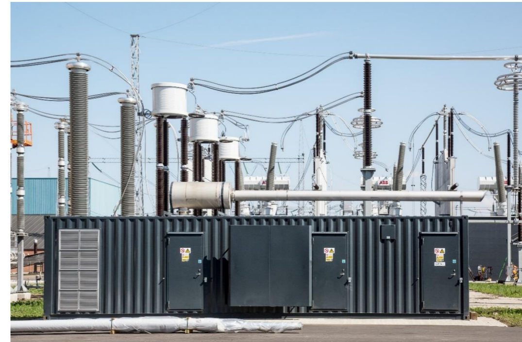
Plate 5.13 – Typical Diesel Generator Image: ©ABB
