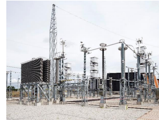
Plate 5.8 – Typical Lightning Masts Image: ©GE
