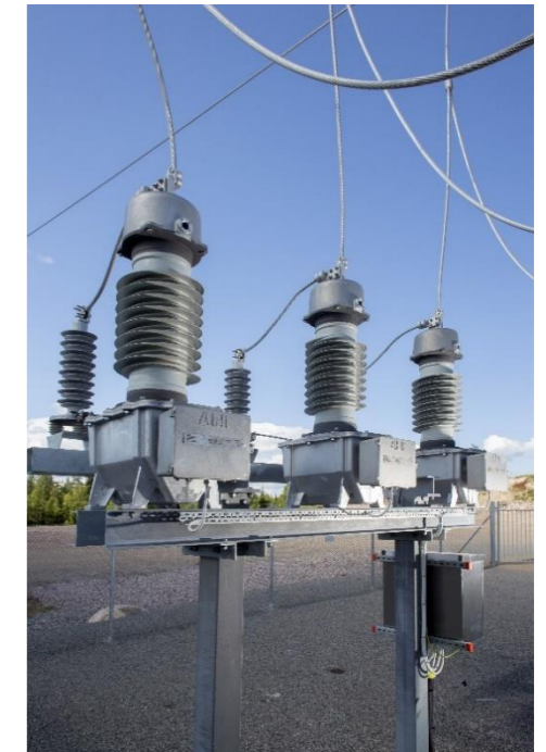
Plate 5.16 - Typical Voltage Transformer Image: ©ABB
