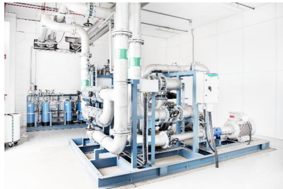
Plate 5.22 – Typical Water Pumping Station Image: ©ABB
