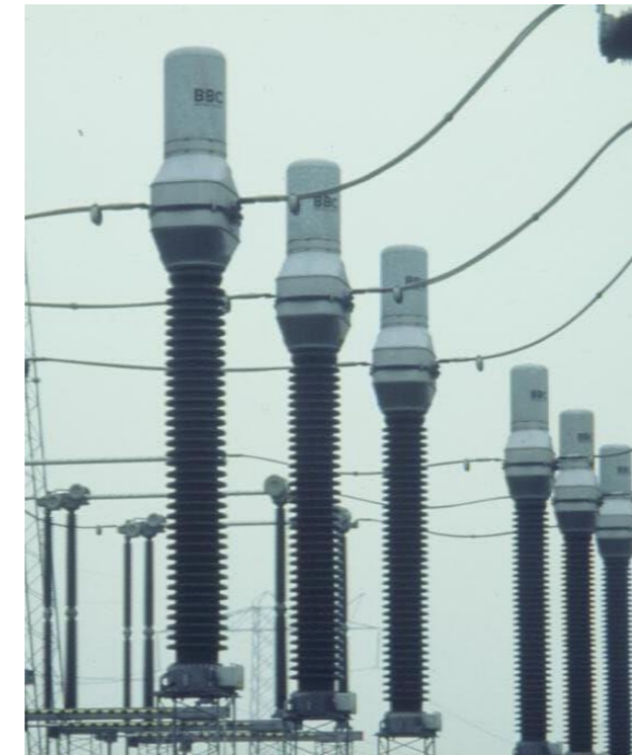
Plate 5.15 – Typical Current Transformer Image: ©ABB
