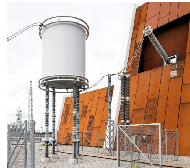
Plate 5.19 – Typical Phase reactors (outdoor) Image: ©GE
