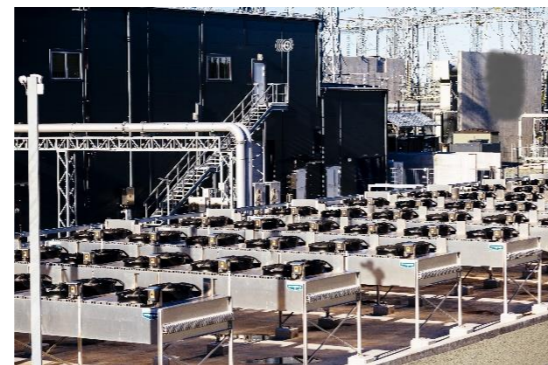
Plate 5.23 – Typical Outdoor Heat exchangers Image: ©GE
